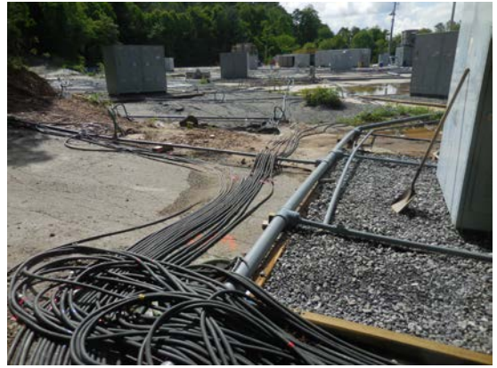
Additional cables and other electrical transformers and control units across source area.
