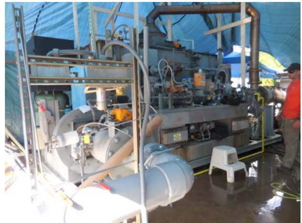
Thermal oxidizer unit and influent piping.
