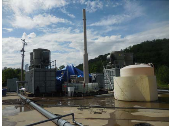
View of treatment system components (note thermal oxidizer exhaust stack in center of photo)
