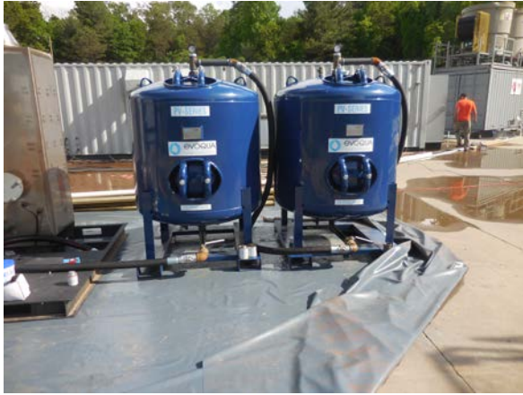
Carbon treatment units.
