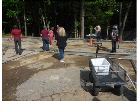
System installations along the eastern property boundary.
