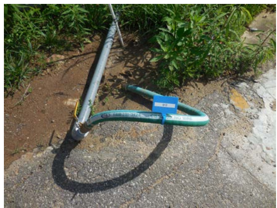
Close-up of recovery piping
