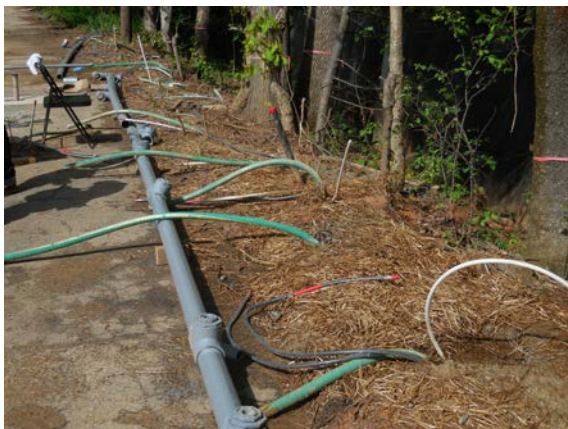
Vapor recovery and electrode installations angled beneath adjacent private property to the east of CTS site.
