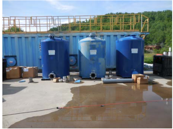
Additional carbon treatment units and water holding tank.
