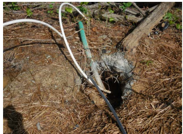
Close-up of vapor recovery and temperature monitoring point installation along eastern property boundary
