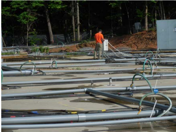
Vapor recovery piping looking toward eastern property boundary.
