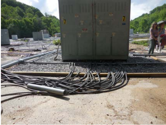
Electrical transformer – one of several -- and incoming cables from electrodes.
