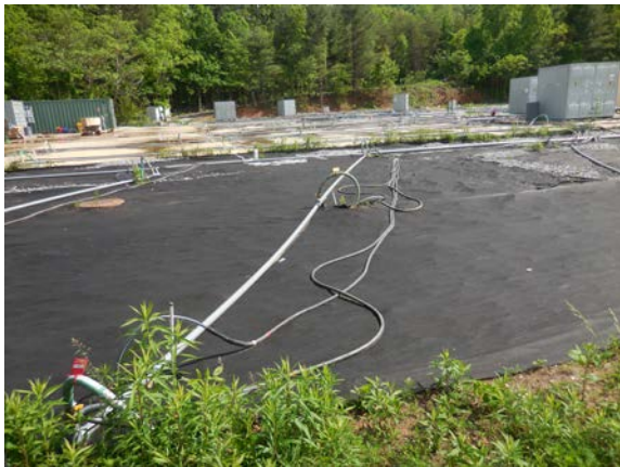
Surface installations including cables, piping, vapor recovery and electrical control units across the 1.2-acre Source Area.
