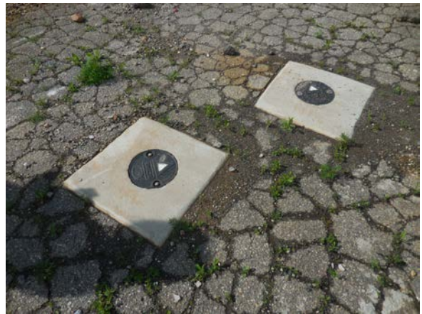
Injection and monitoring wells where ISCO potassium permanganate was injected.
