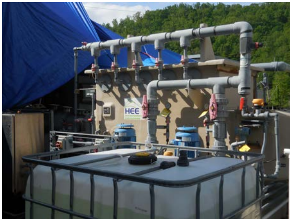
Vapor recovery system manifold at treatment system for metering vapors into thermal oxidizer where TCE and VOCs will be destroyed.
