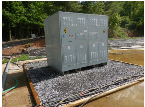
Electrical transformer (one of several as the system is zoned to enable optimization of remedial action).
