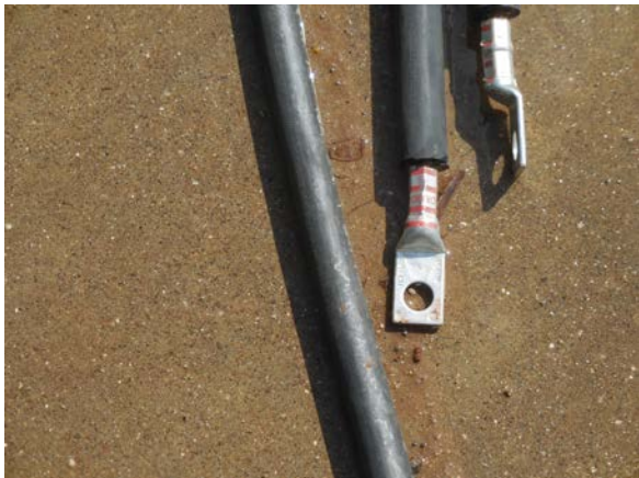
Close-up of electrical cable connection fittings for attachment to electrodes.
