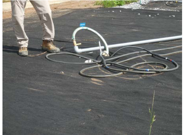
Close-up detail at electrode and vapor recovery well head. Note electric cable and vapor recovery piping.
