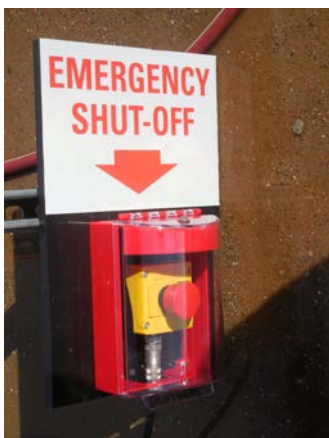
Emergency shut off control at thermal oxidizer. System has integrated monitoring with auto-shut off in case of higher-than allowed VOC exhausts.
