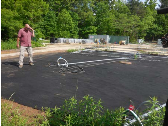
EPA's Mr. Zeller at the Source Area of CTS Superfund Site, south side of Mills Gap Road. Note impermeable cover over treatment area.
